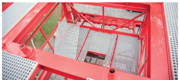
Injector platform with centering bolts
