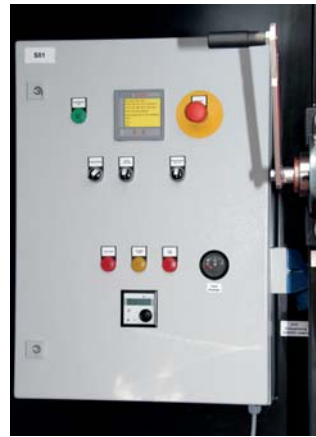
Electric control panel
